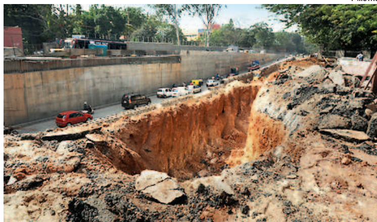
BBMP approved the underpass in 2008, but work is still on, says Rao (above right)
